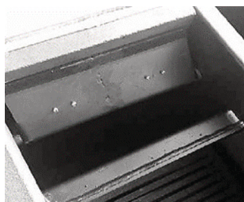
Closed flue gas deflector (17)
