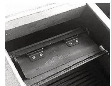
Open flue gas deflector (17) ⇒ Boiler efficiency significantly reduced!
